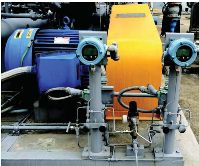
Pump Emergency Shutdown
